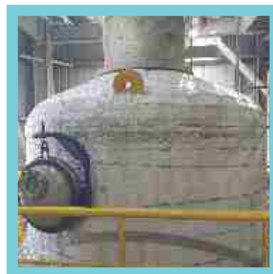
Perlite block on Equipments
