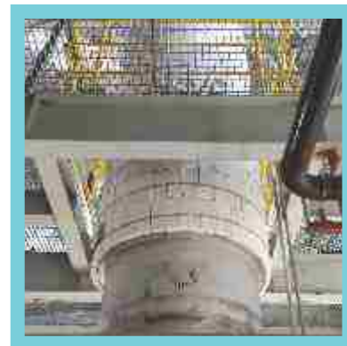
Perlite Block on Large Piping
