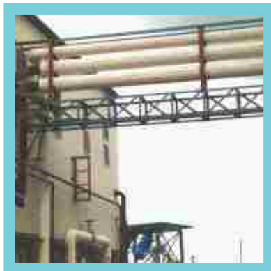
Straight pipe section
