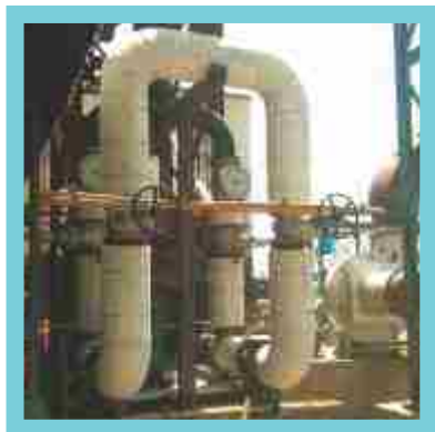
U-Loop Pipe Section
