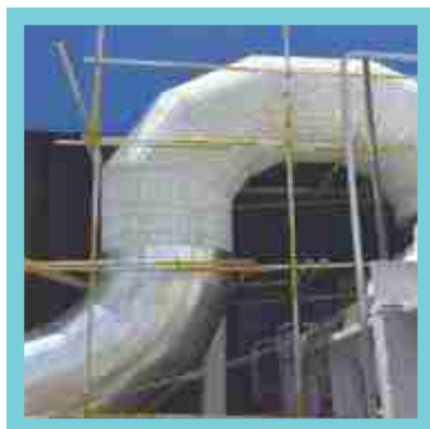
U- Bend big piping-by Perlite block
